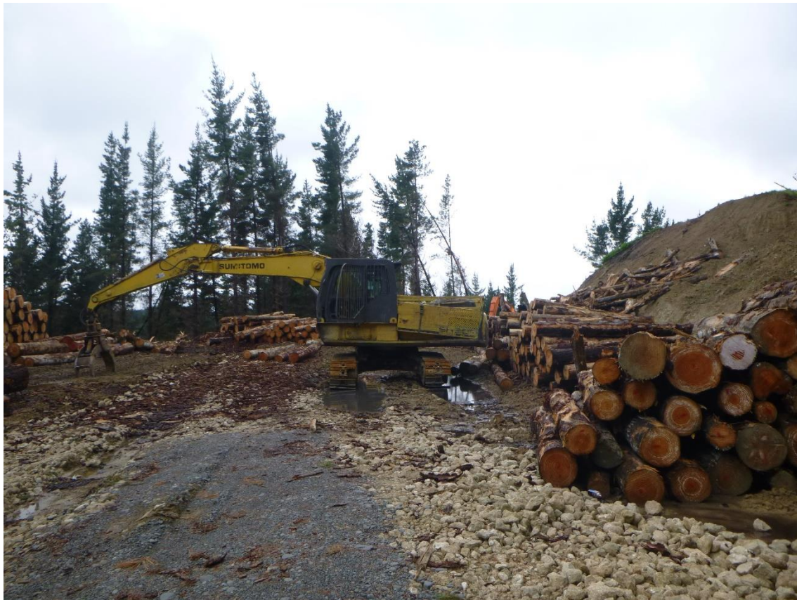
Photo 1: A very wet Landing 31 following Cyclone Gabrielle.
