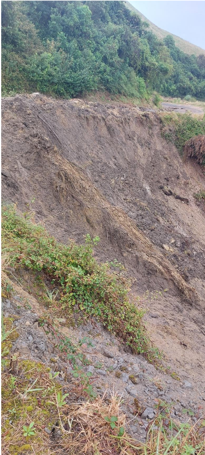
Photo 3: Dropout at Marker 14, Putere Road.
