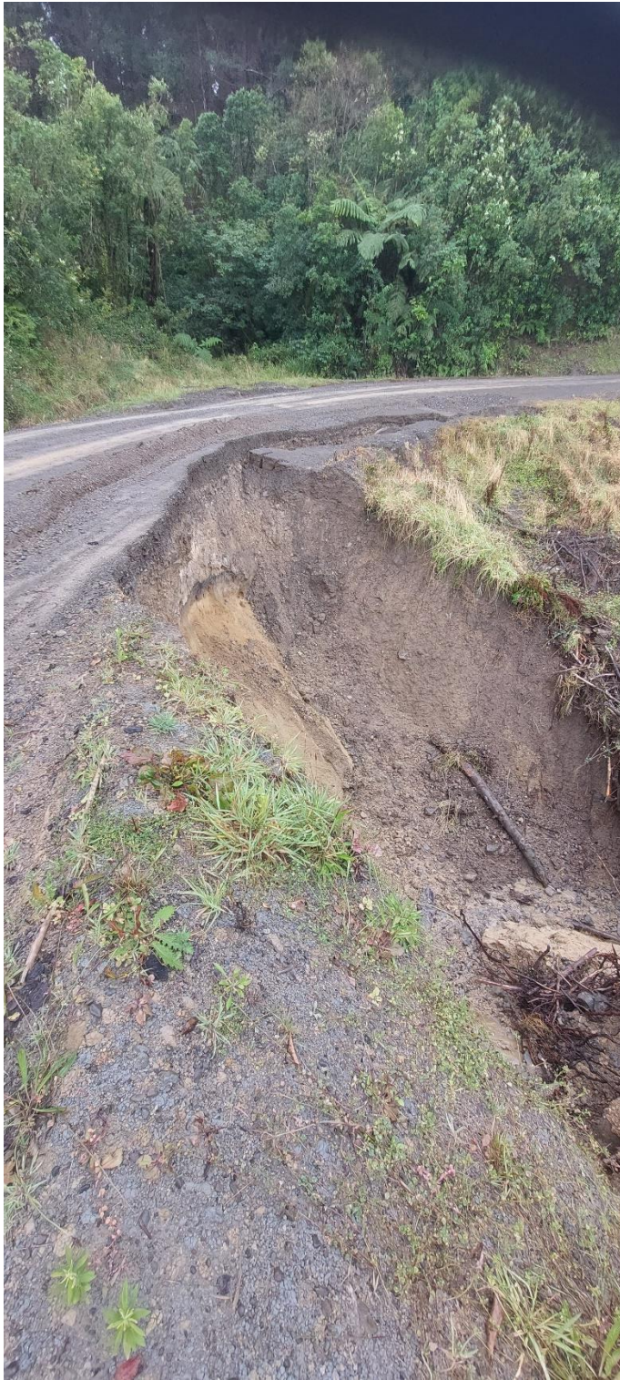
Photo 1: Dropout at Marker 8, Putere Road.
