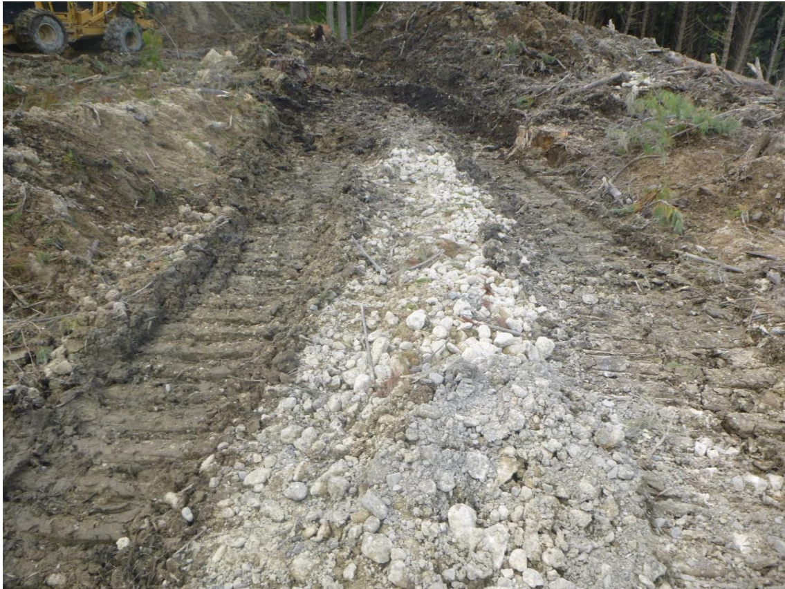
Photo 5: Loadout bay failing due to soft ground conditions at Pad T2.
