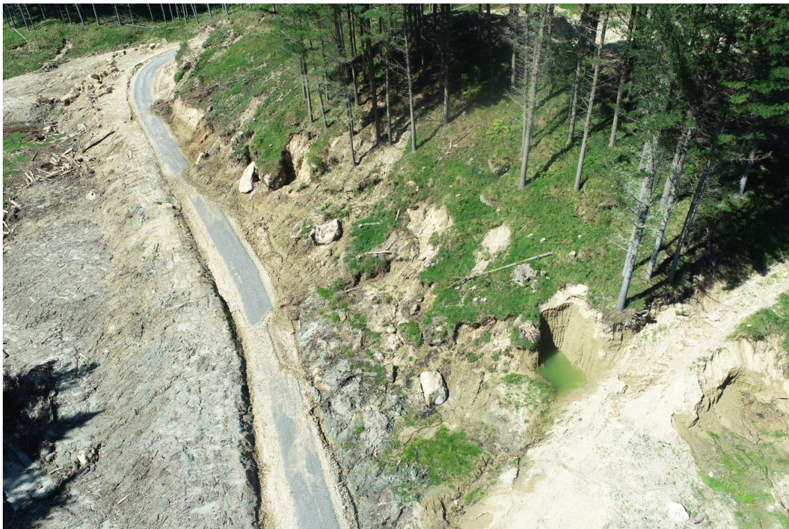
Photo 4: Slips and damage to water controls on Griffiths Road.
