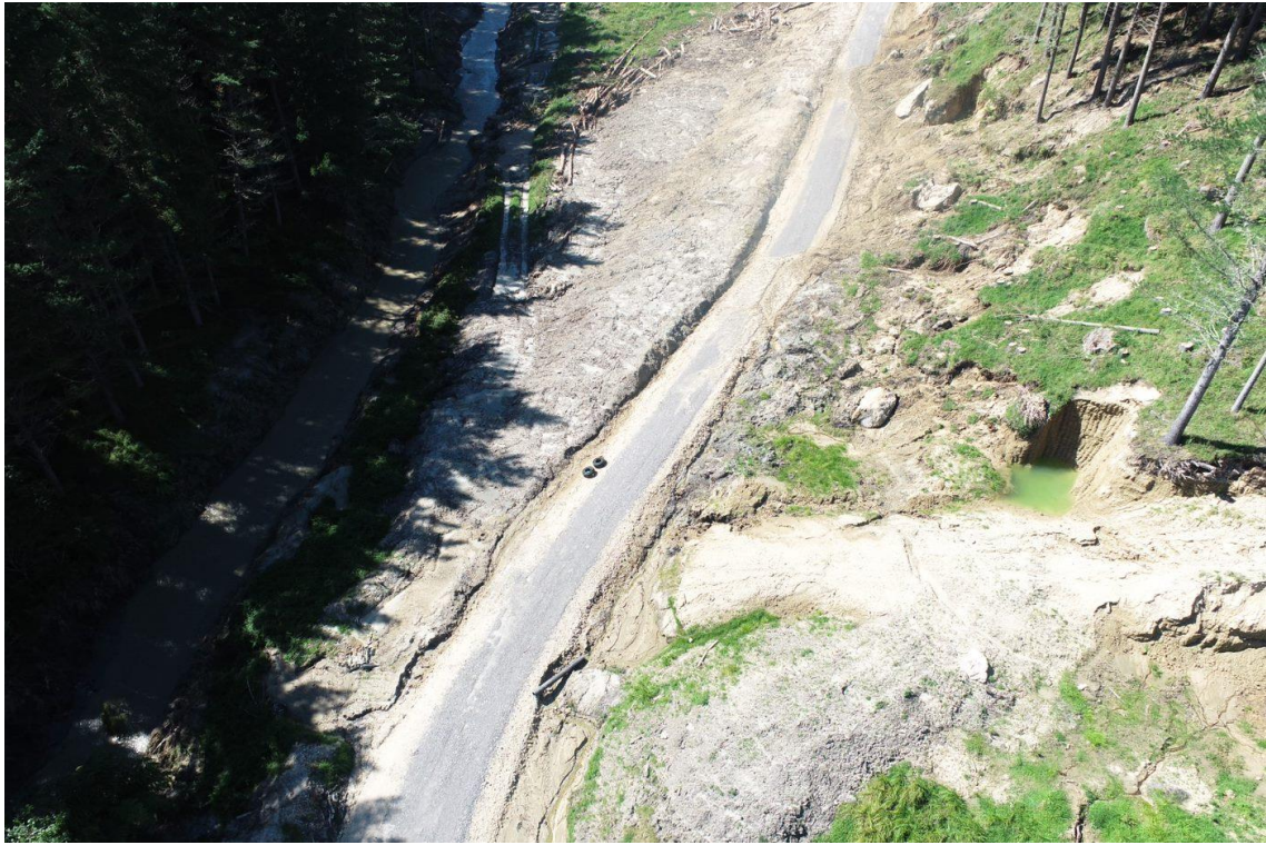
Photo 5: Track damage on Griffiths Road.
