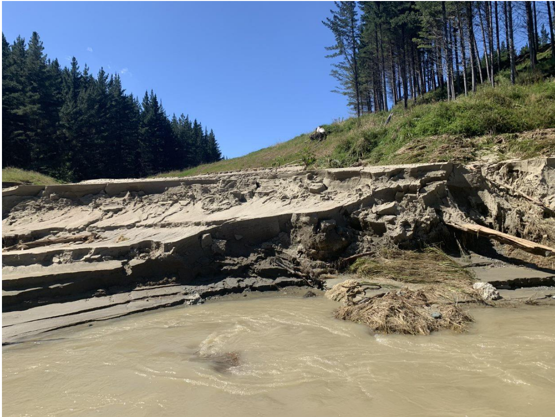
Photo 1: Cyclone damage to low level crossing on Griffiths Road.
