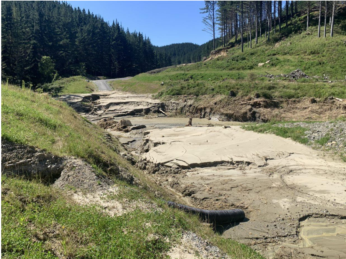
Photo 3: Further damage to low level crossing on Griffiths Road.
