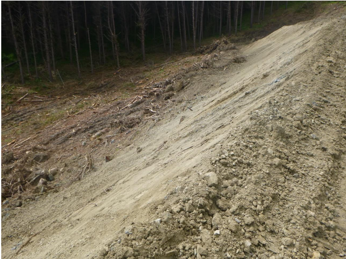
Photo 3: Fill material contained on a bench below White Road.
