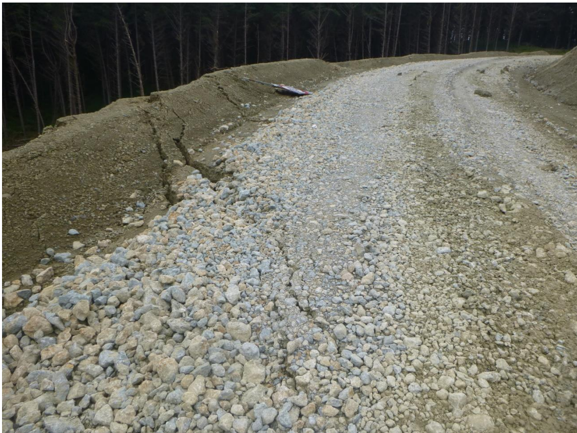
Photo 18: Cracks on Mad Mutt Road following cyclone Gabrielle.
