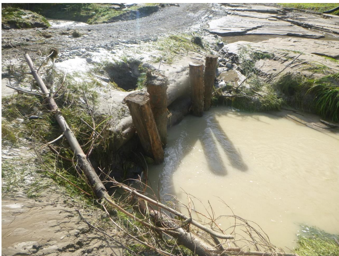
Photo 20: Damage to the temporary crossing at the 3km marker on Mad Mutt Road following cyclone Gabrielle.
