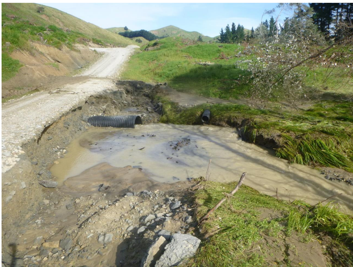
Photo 19: Damage to the temporary crossing at the 3km marker on Mad Mutt Road following cyclone Gabrielle.
