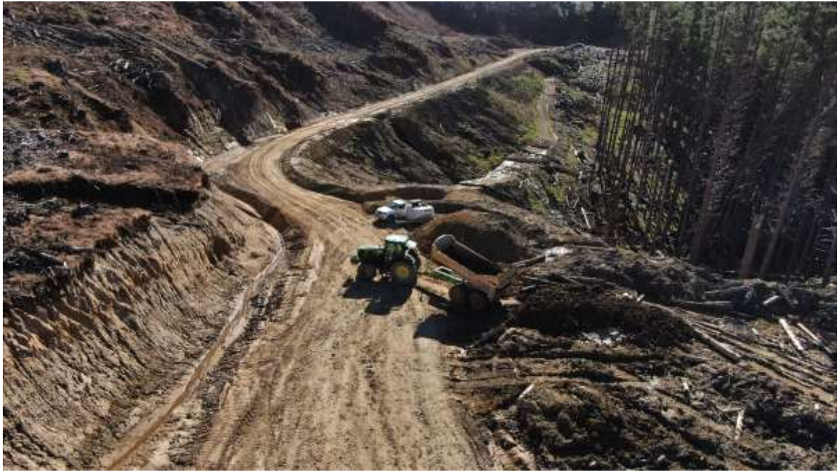
Photo 3: Setting 500, a section of road reopened after March storm events.
