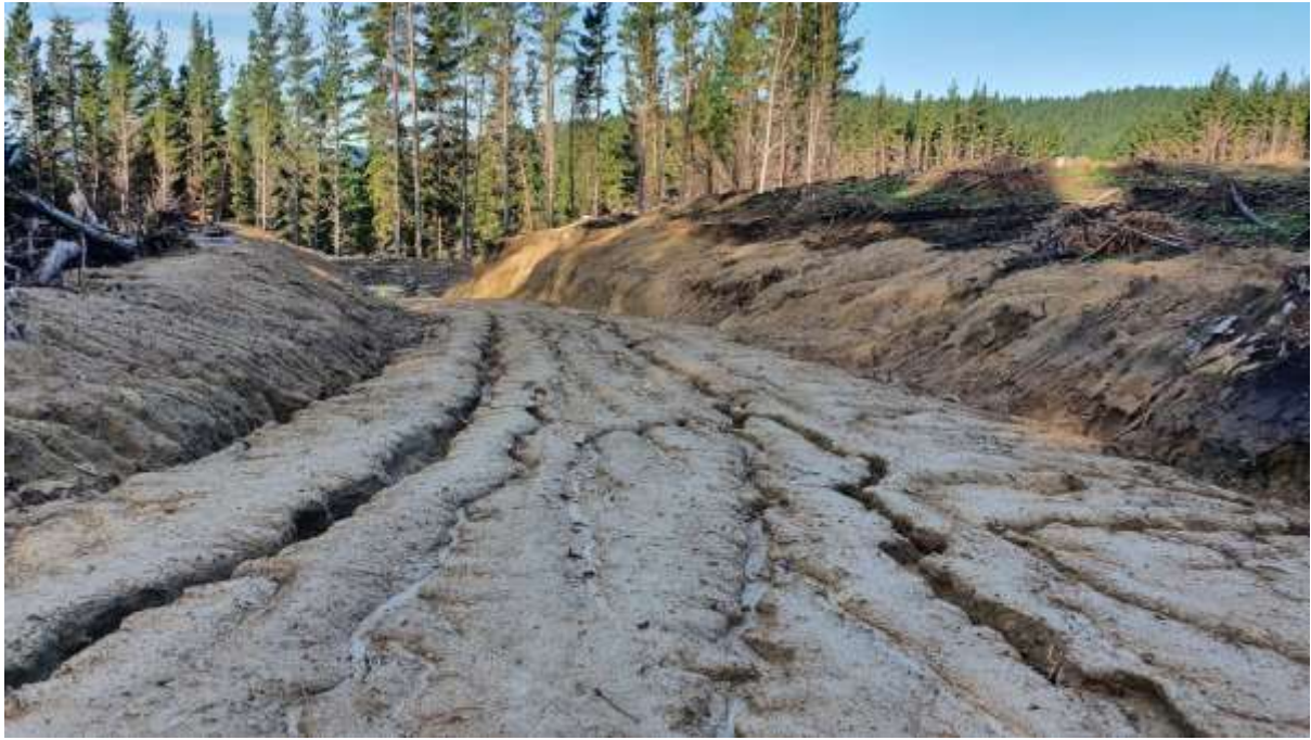
Photo 1: Setting 500 two-stage track sustained rilling after storm event requiring controls by maintenance crew to avoid loss of infrastructure.
