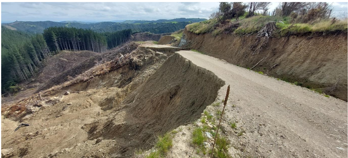
Photo 2: Large dropout on Cardiff Road.
