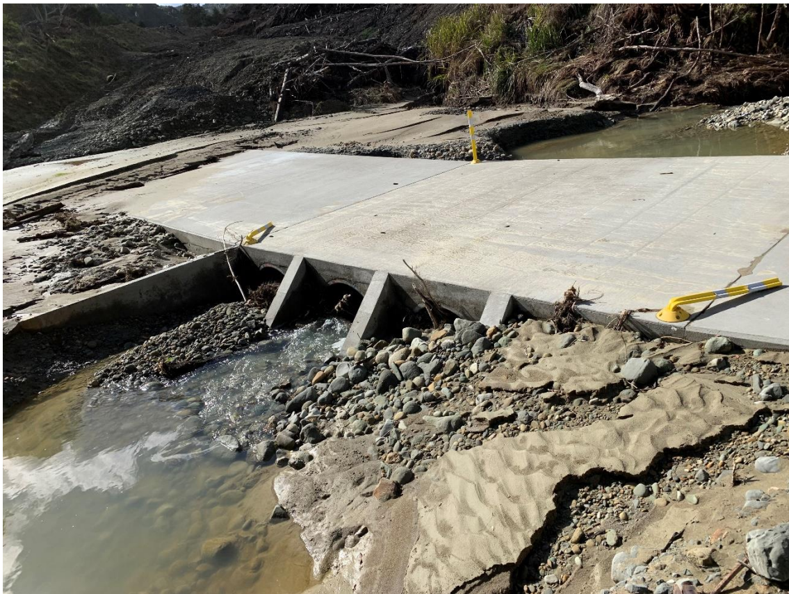
Photo 2: Culvert crossing after large heavy rainfall event.
