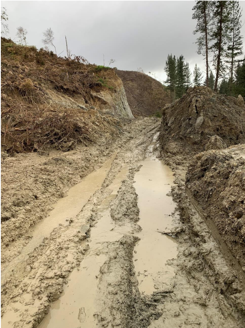
Photo 3: Section of McCoy Road between markers G7 and G8 after large heavy rainfall event.
