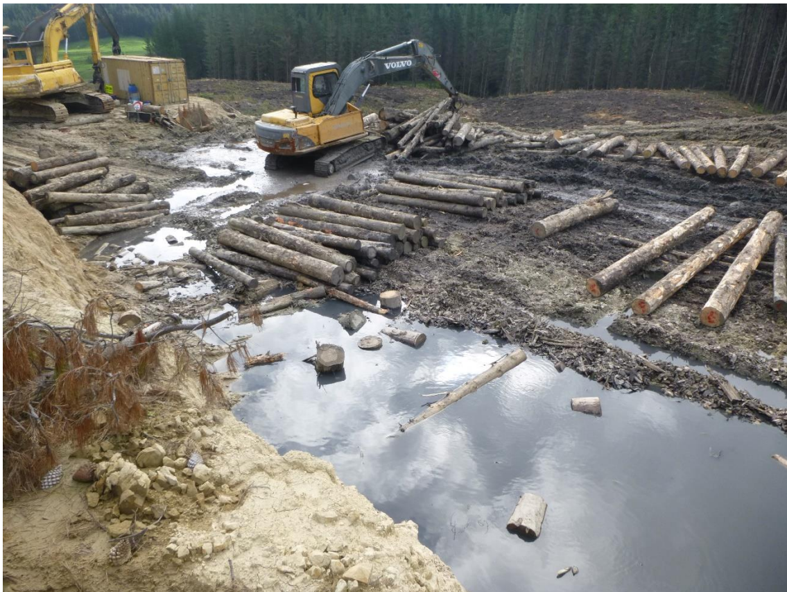
Photo 2: A very wet Landing 4.
