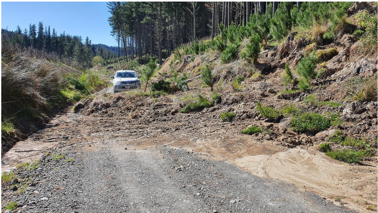
Photo 4: Failed slope blocking Black Road after storm event, requiring maintenance machine to clear to allow vehicle access.
