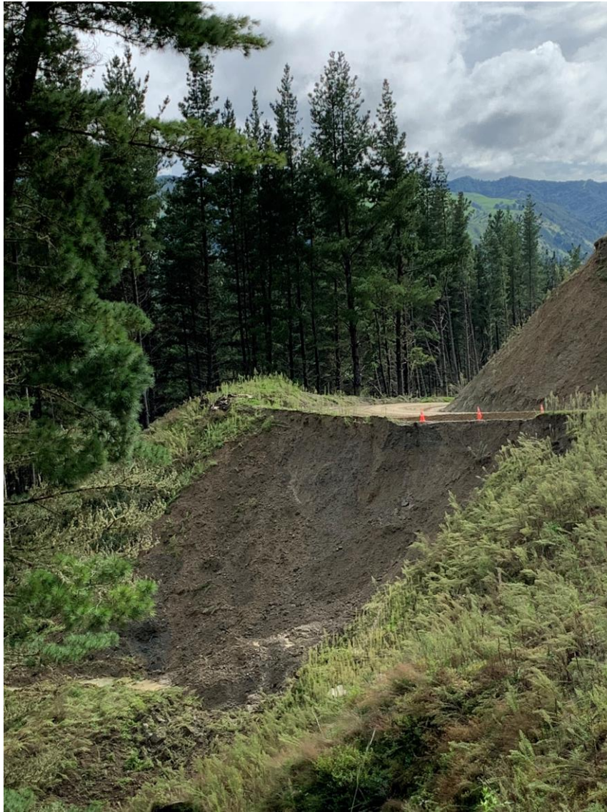
Photo 2: Richmond Road dropout at Marker 4.
