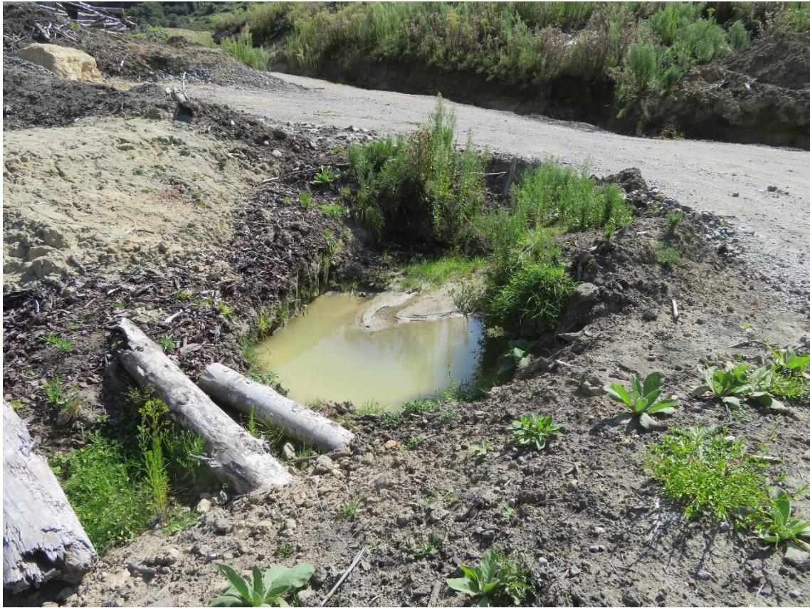
Photo 4: Sediment trap used for treating stormwater discharge.
