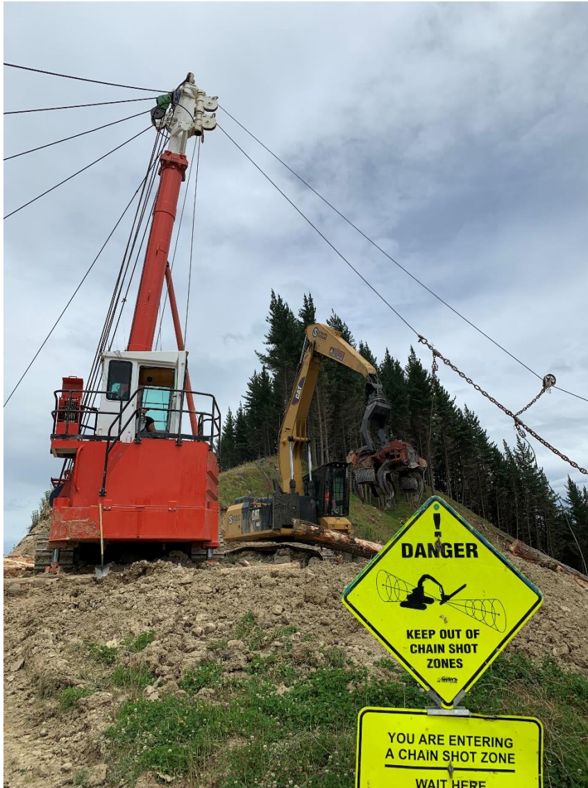
Photo 3: Hauler zone with warning signs.
