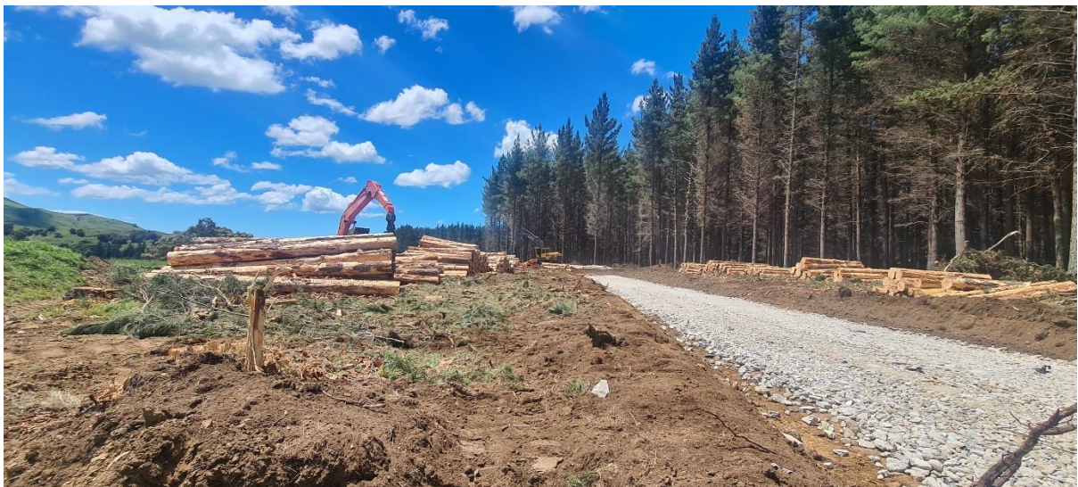
Photo 2: Rolled end of Tutaekuri Road near temporary landing.
