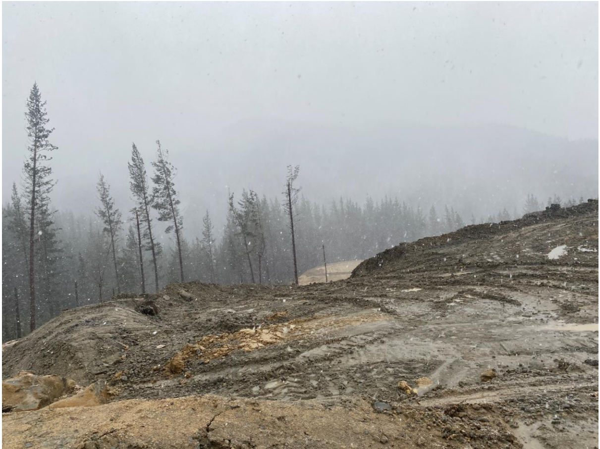
Photo 6: Snow storm coming in on Landing 43.
