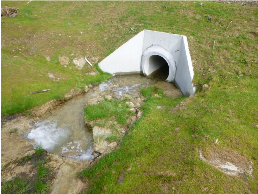
Photo 3: Water flowing through Crossing 4 on Rolfe Road with the results of earlier grass seeding visible with strong grass growth.
