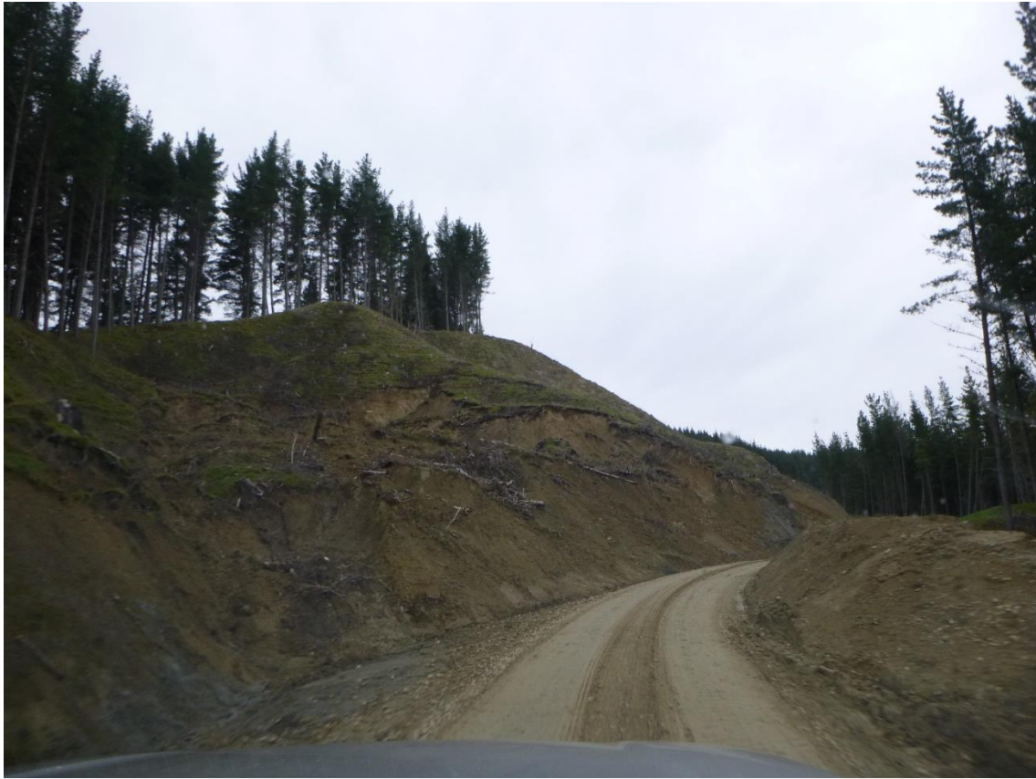
Photo 3: Instability of batter slope at Marker 2 on Richmond Road.
