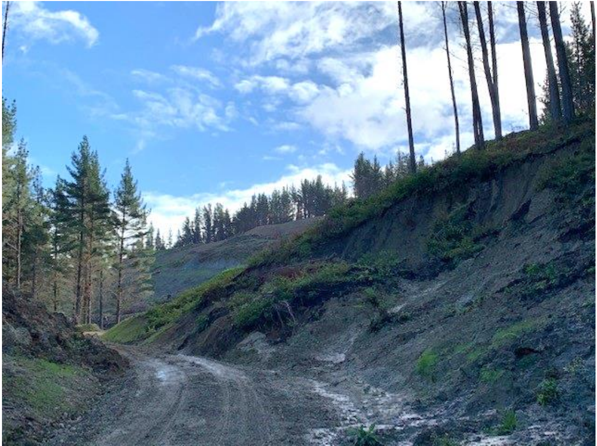
Photo 1: Slip on Cairns Road from heavy rain event.
